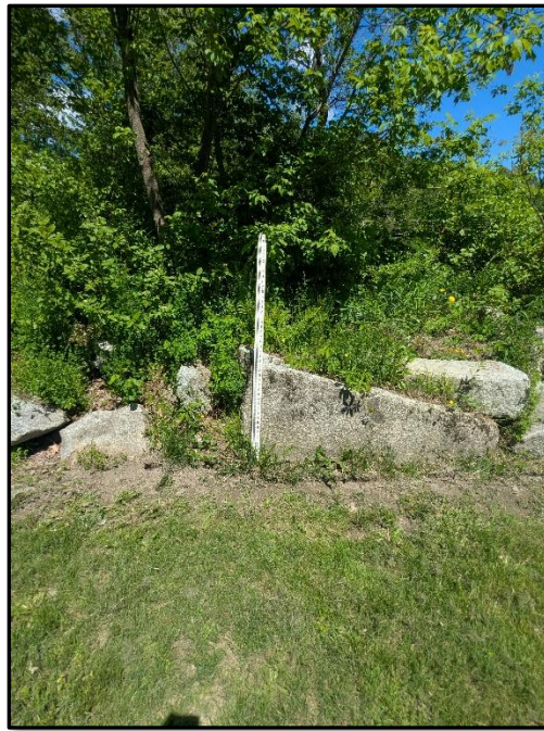
Photo 5. Large riprap along the right bank just upstream of the Rte 105 bridge. The riprap was placed along the right bank when the bridge was constructed (see Photo 2a.)
