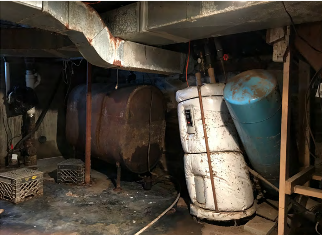
furnace, water heater, pressure tank destroyed, oil tank must be replaced
