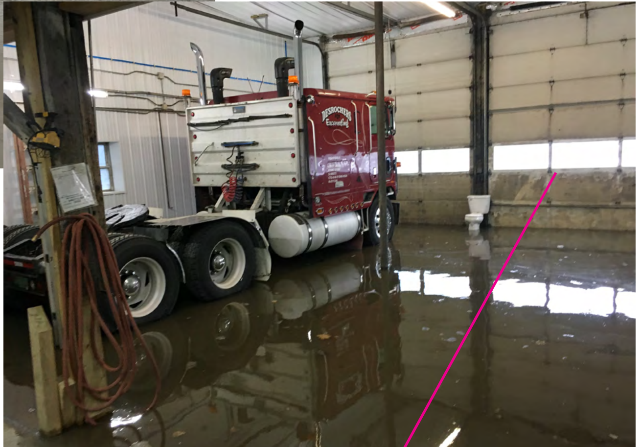
Note high water crested mark during January 13, 2018 Inside garage bay after most of water has subsided January 2018
