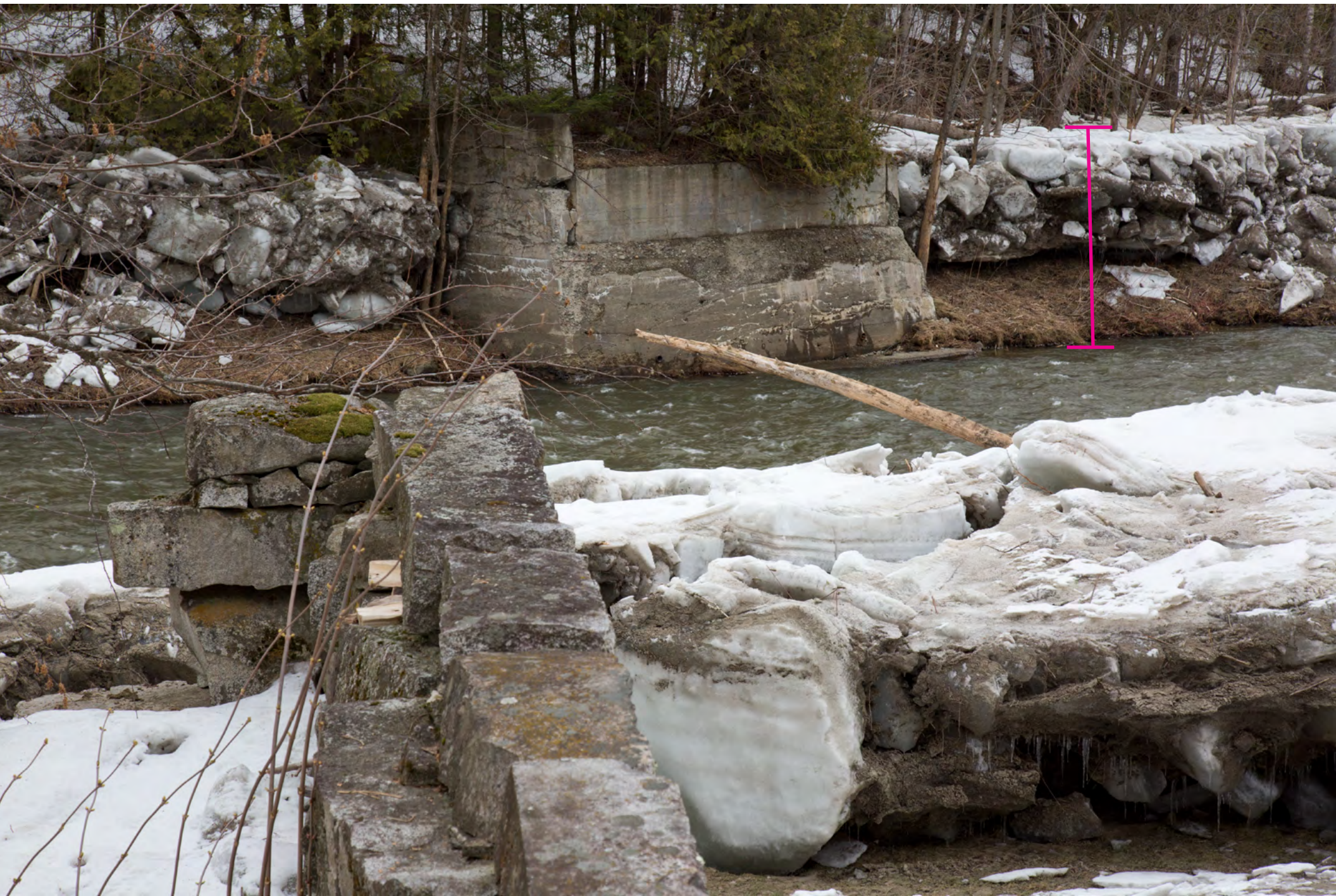
mid-April 2018 Grist mill foundation in foreground Note height of ice jam to right of bridge abuttment (approx 15 feet) 3 months after ice jam
