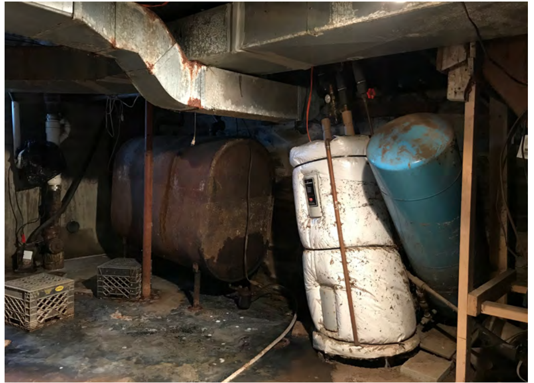
furnace, water heater, pressure tank destroyed, oil tank must be replaced
