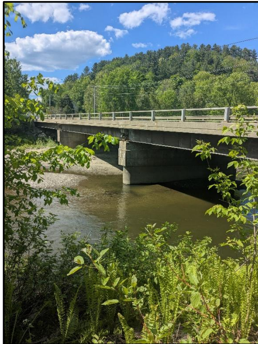
Photo 4. Looking at the Rte 105 Bridge from the right bank towards the left bank
