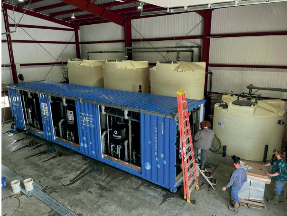
SAFF Unit Inside the Leachate Pre-Treatment System Building
