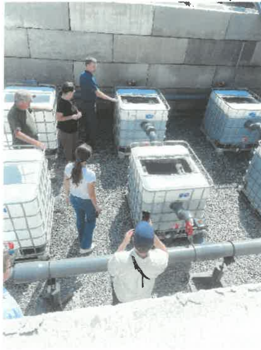
Underdrain Groundwater Treatment System
